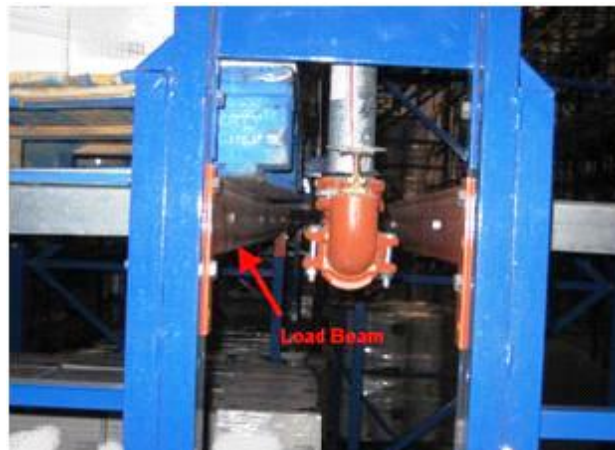
Figure 6.: In-Rack Sprinkler Position.
